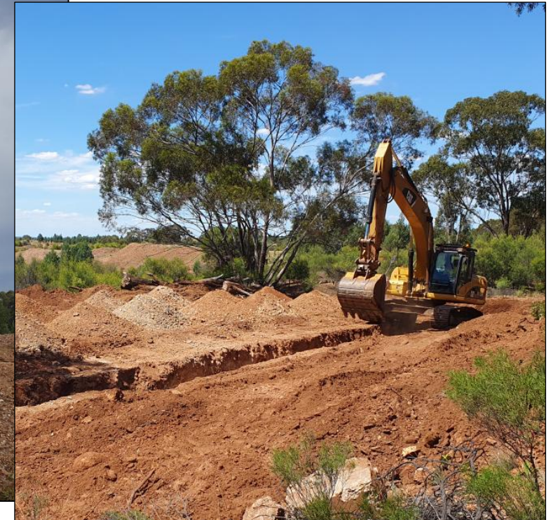
Trench T5 while being excavated – looking north towards the edge of the Southern Open Pit with the walls in background
