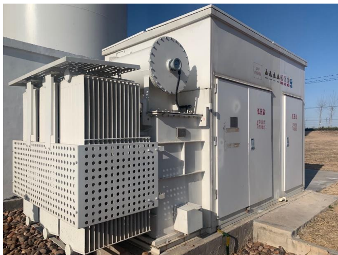
5500kVA wind power step-up amorphous transformer
