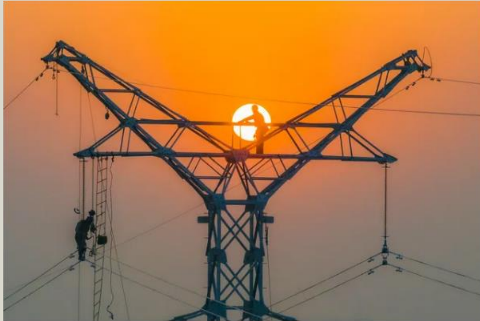
Workers erect a steel tower at the 220kV line project in Jiangsu Province, China, on October 16th, 2023. Photo by Costfoto / NurPhoto via Getty Images
