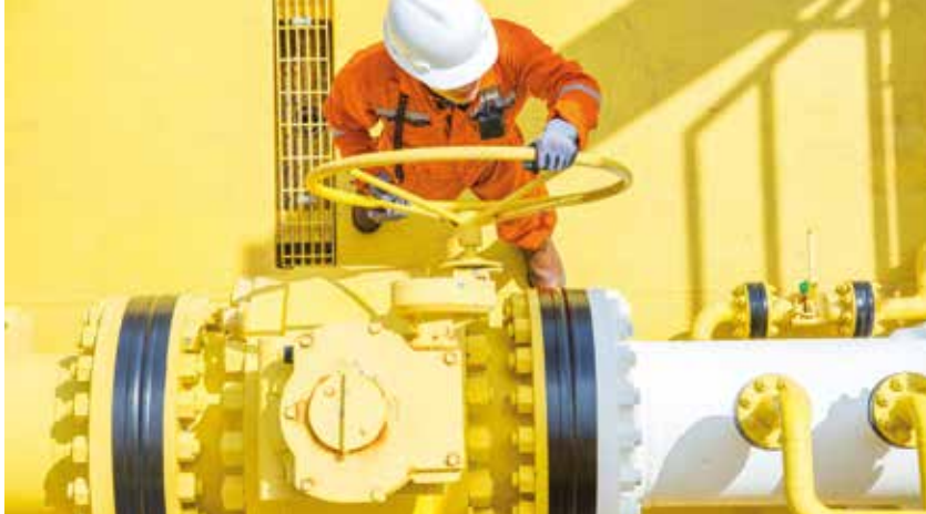
An ADNOC technician turns valve wheel on a pipeline system in Abu Dhabi. Credit Shutterstock
